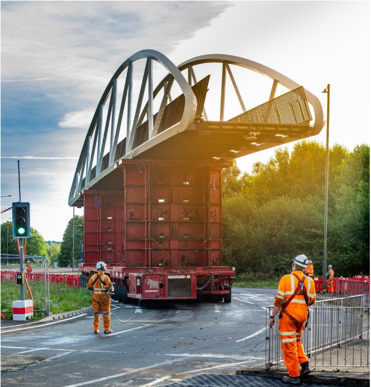
4. Bridge being transported into place on a self-propelled modular transporter unit from the site welding compound adjacent to the road
