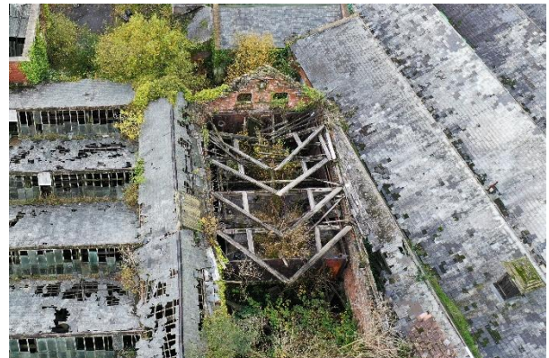
Figure 1 The tank was obscured by the collapsed roof trusses, debris and vegetation
